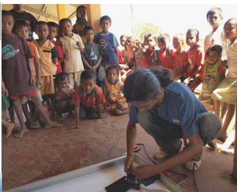
Timorese trainee installs solar panels in a Maliana school – under close supervision
